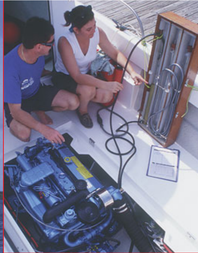
F&B's Ruth Cunningham monitors the Nanni diesel's fuel consumption with Arvor Queensland agent Ray Bride. Note the excellent access right around the Nanni for easy servicing and daily checks.
